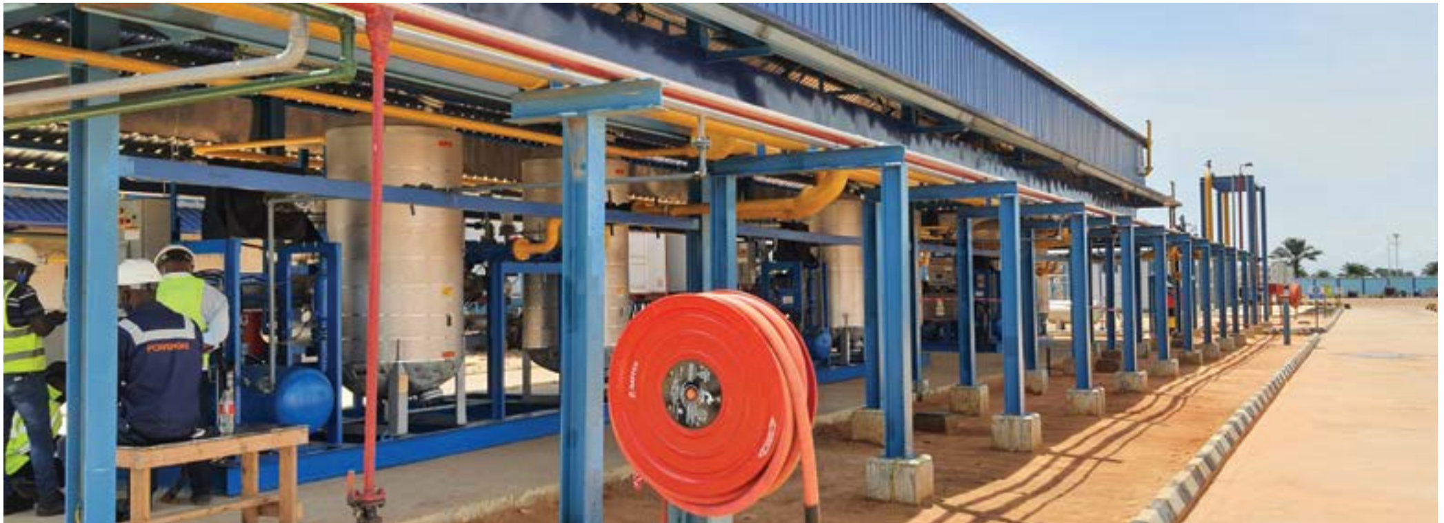
IMPALA CAPTIVE POWER PLANT
